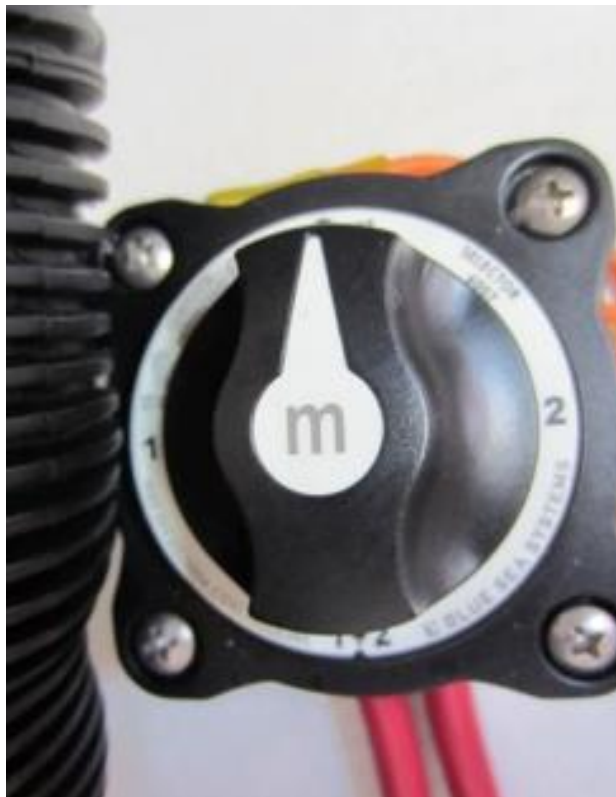
Battery Switch, Shown in the “Off” Position
