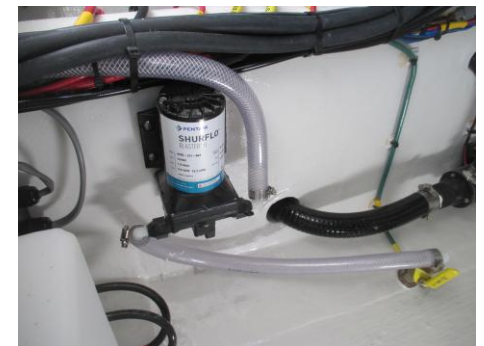
Saltwater Pump & Intake Valve
