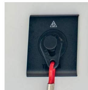
Engine Stop Switch
