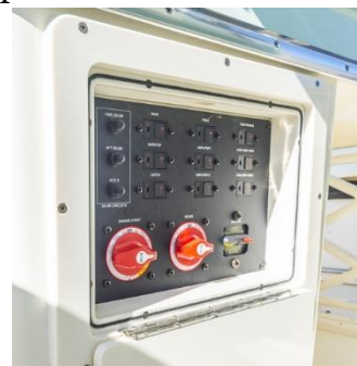
Battery Switch (Shown in the Off Position)
