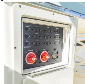
Battery Switch (Shown in the Off Position)
