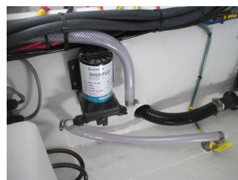
Saltwater Pump & Intake Valve
