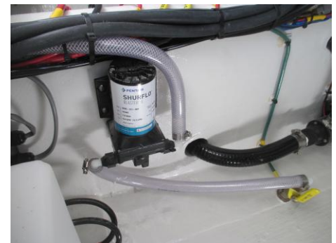
Saltwater Pump & Intake Valve
