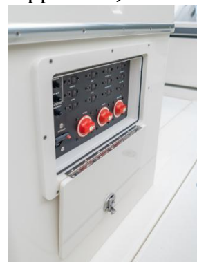
Battery Switch Panel
