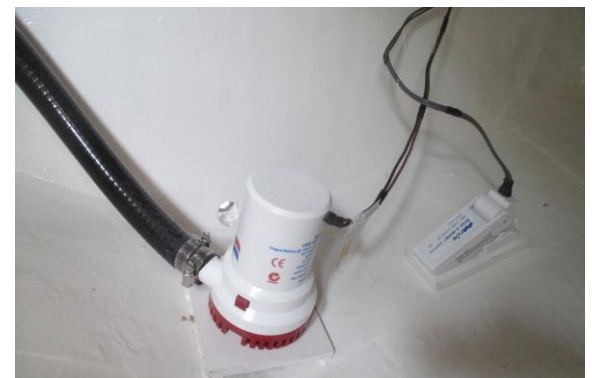
Aft Bilge Pump and Float Switch
