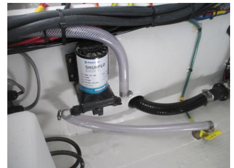
Saltwater Pump & Intake Valve
