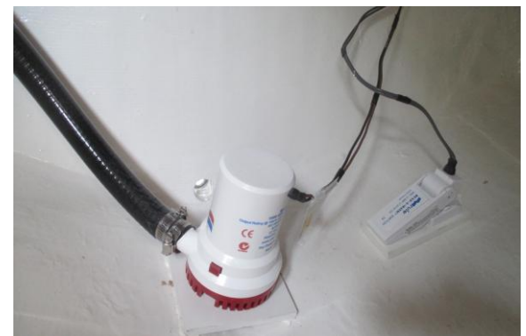
Aft Bilge Pump and Float Switch
