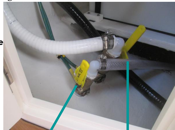
Intake Valve (open)
