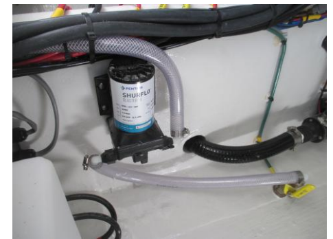
Saltwater Pump & Intake Valve
