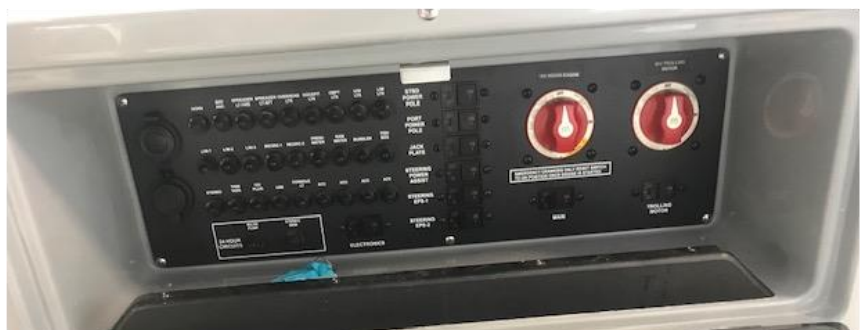
Battery Switch, Shown in the "OFF" Position
